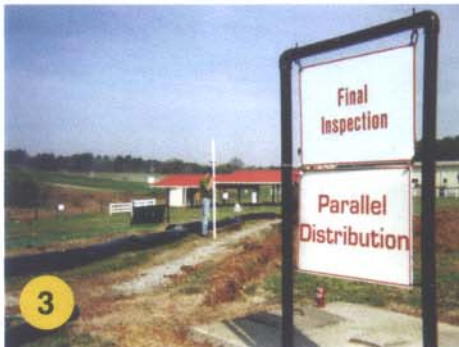
3 Laser Level check of trench depth grade and bag encased protected pipe moved onto trench site. The plastic bags protect the filter wrap from extended storage UV deterioration and natural handling abuses.
